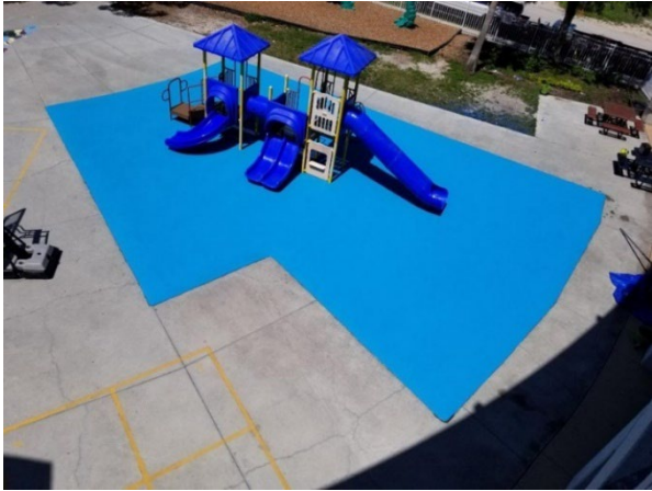
Image 1: A floor covering made of light blue rubber granules installed with an aromatic binder directly after installation.
